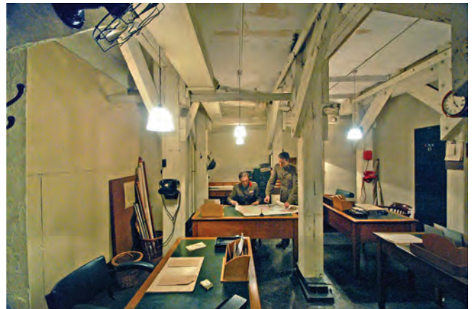
Timber framing in the Room 62A of the Cabinet War Rooms possibly installed as part of the late 1940s strengthening works when a reinforced concrete slab was inserted above the bunker in the New Public Offices' sub-basement. The large square posts rest on spreader wedges and support tripled up bolted joists, on this occasion diagonally braced to resist lateral ground shock movement. Photo from Cabinet War Rooms
